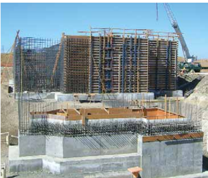
Lower level of headworks with aeration basin in background.
