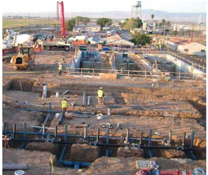
Underslab piping at membrane building slab with the aeration basin in the background.
