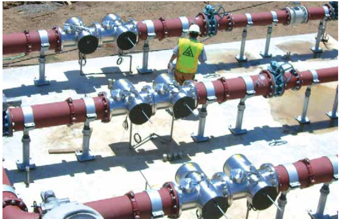
Ultraviolet disinfection piping.
